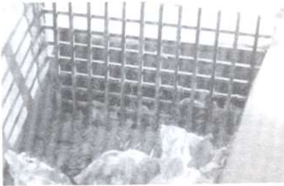
Plastic bags dumped in sewers and drains often cause blockages and resultant overflow.
